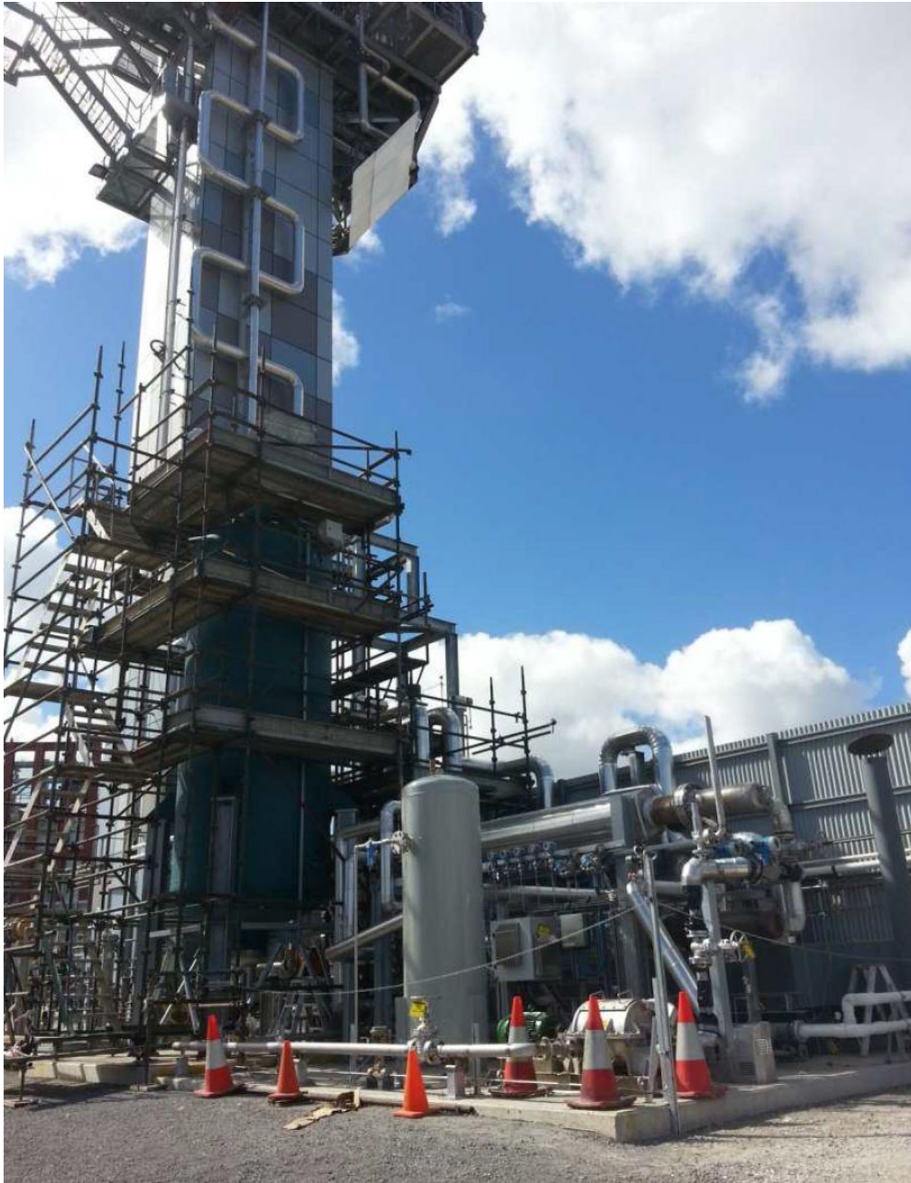
Figure 1 - The completed 750kWh solar thermal energy loop
