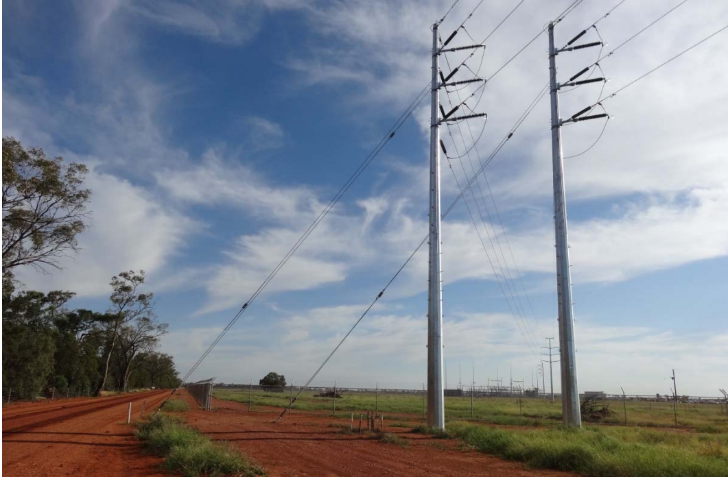
Photo: New 132 kV line at Nyngan
