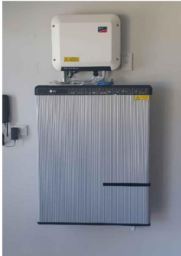
Figure 2. The first VPS2 LG-Chem Battery and SMA Battery Inverter Installation
