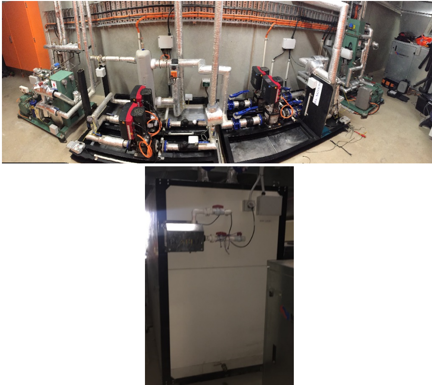
Fig. 2 The 20 kW refrigeration plant and PCM tank at The Bends Motorsports Park.
