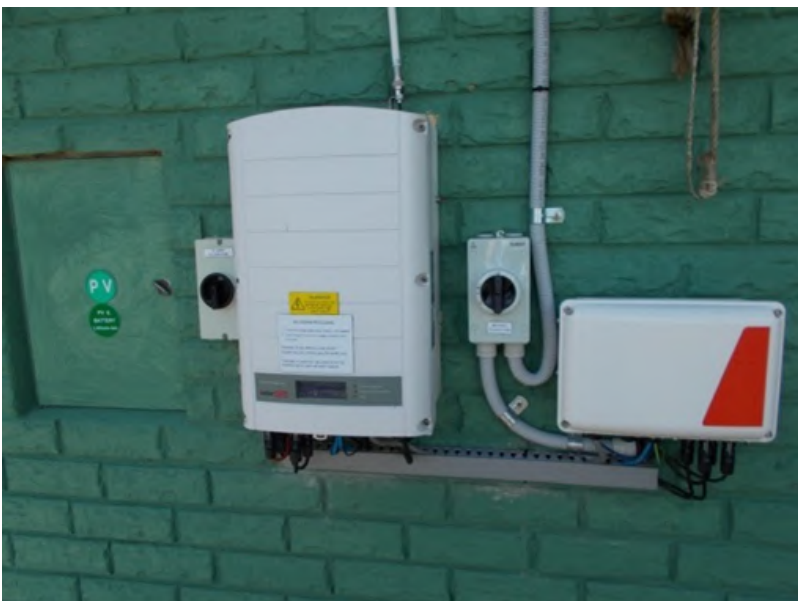
Plate 3: Example of installation with no enclosure
