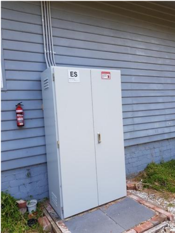
Plate 2: Cupboard enclosing battery equipment (external)
