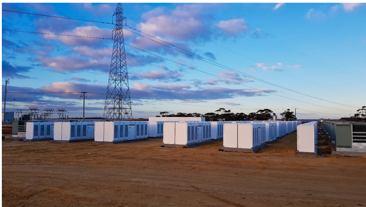
Figure 10 GESS and 220kV AusNet transmission line
