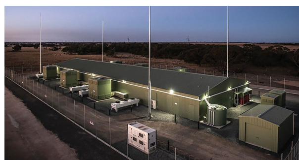
Energy Storage for Commercial Renewable Integration Electranet
