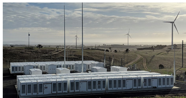
Lake Bonney Battery Energy Storage System Infigen Energy
