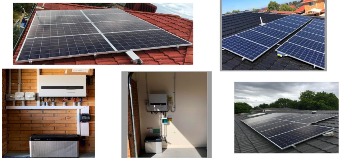
Figure 6: Typical customer installations from United Energy's residential solar and storage program.
