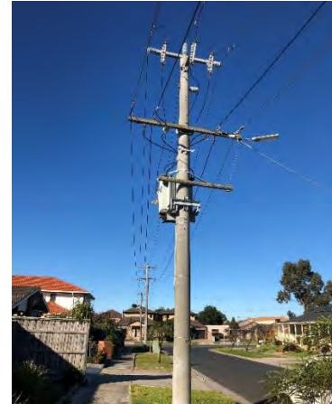
Figure 2.1. A picture of LVDN (only with several poles and the overhead lines)
