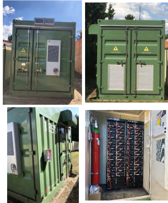
Figure 5.1. Views of the BESS enclosure
