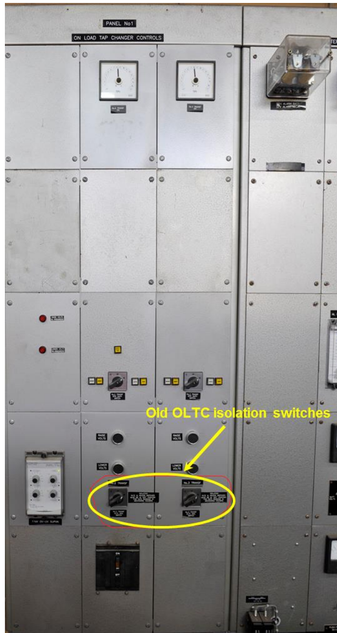
Figure 8 OLTC isolation switches utilised by legacy MD3311 OLTC RTUs
