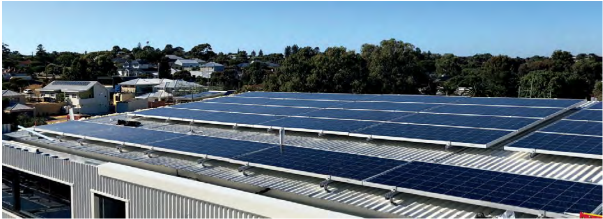
Figure 11 Evermore solar PV mounted on roof.
