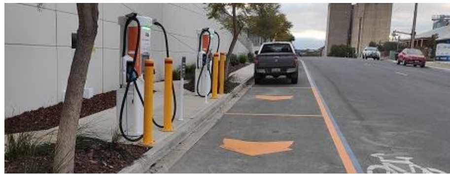
Figure 12: Chargefox Murray Bridge.
