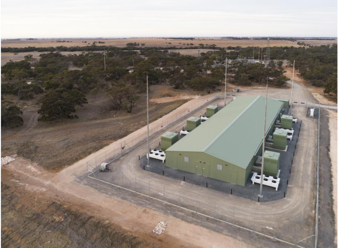
Figure 2-1: Aerial photograph of Dalrymple BESS and the Dalrymple substation looking south
