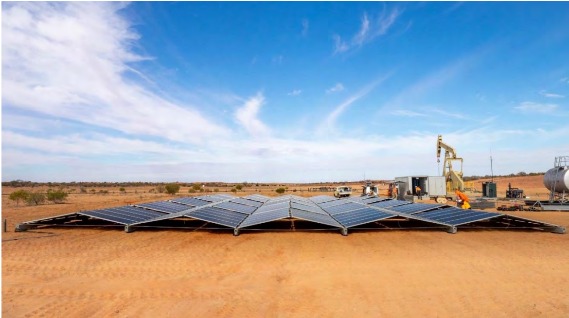
Figure 1 – Solar Installation at Stimpee 1
