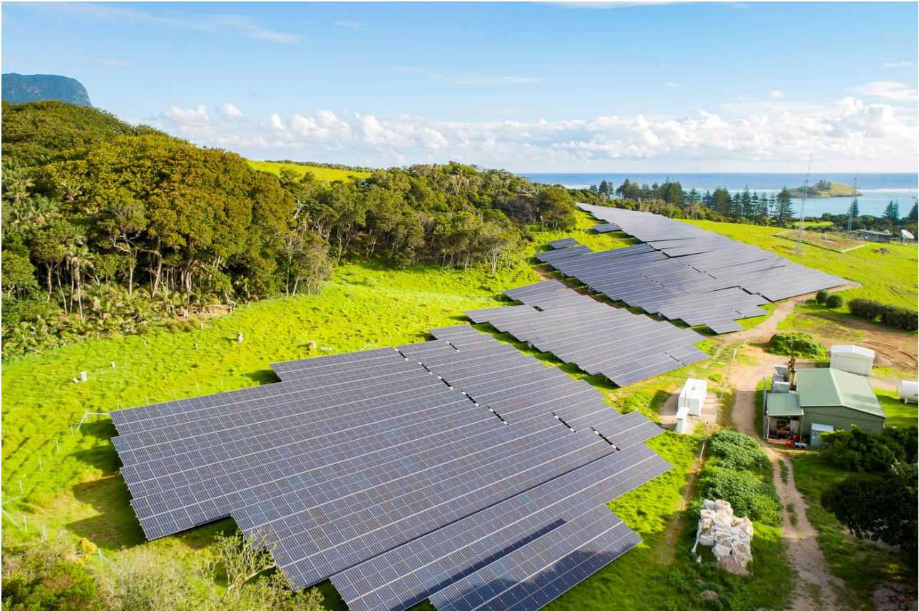
Figure 1-1 HREP solar array, BESS (white container) and powerhouse (green shed)
