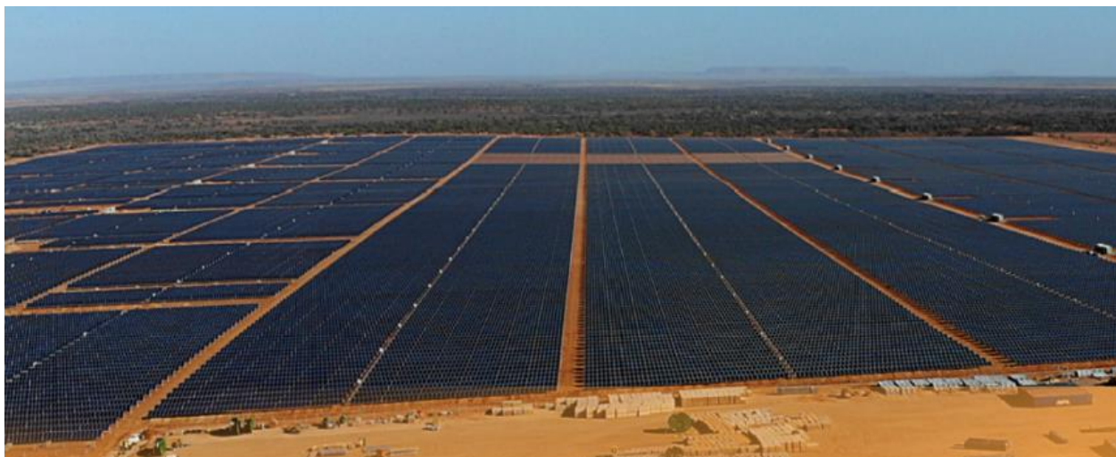
Figure 16 A large scale solar PV farm
