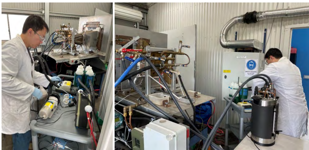
Figure 1. The integrated 1 kW PVE system. (Dr. Jian Pan was operating the alkaline water electrolyser stacks in the images)
