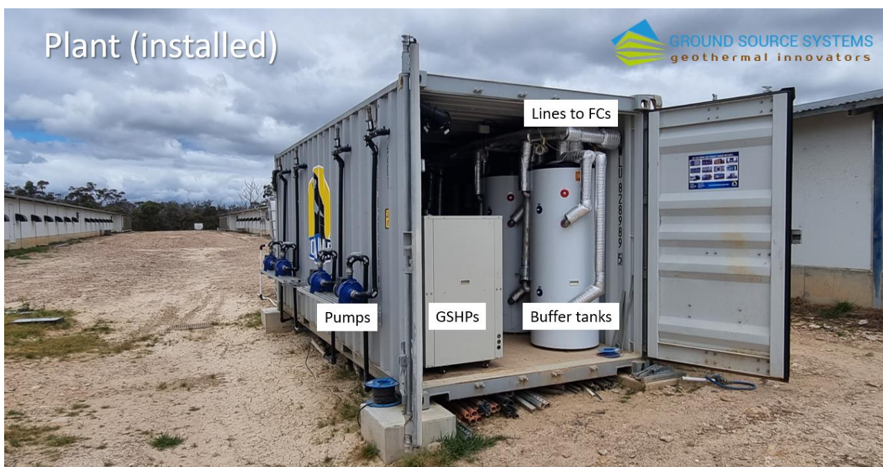
Figure 1. Plant comprising of circulation pumps, ground source heat pumps (GSHPs), buffer tanks, control (and monitoring) systems. Insulated pipes connected to fan coil units (FCs) inside the demonstration shed (right) completes the system.
