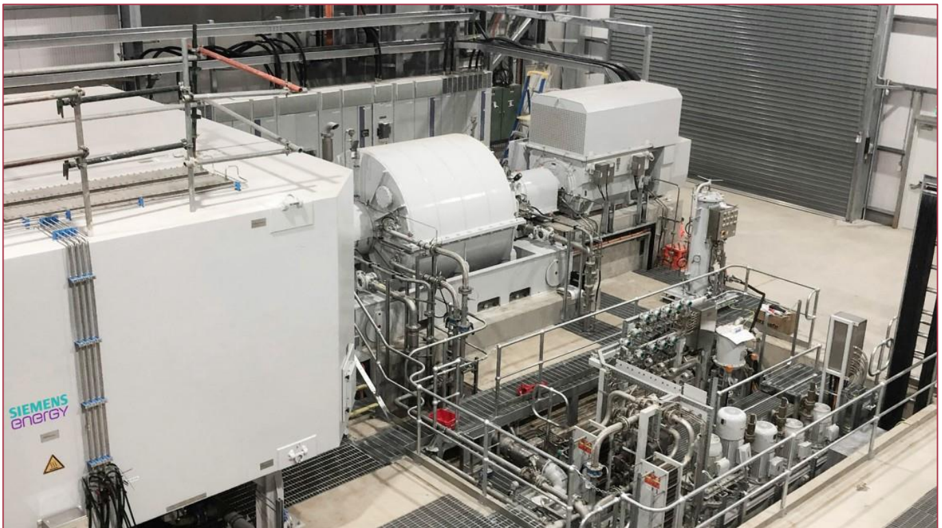
Figure 4.2: Example of a Siemens flywheel installation between a purpose-built SC (left) and the pony motor (right) [8]
