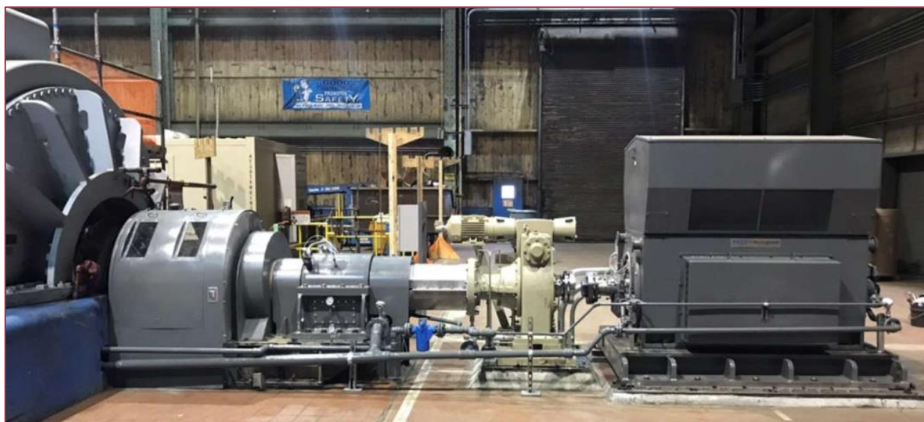
Figure 4.1: Synchronous condenser arrangement with pony motor on right and synchronous machine on left [7]
