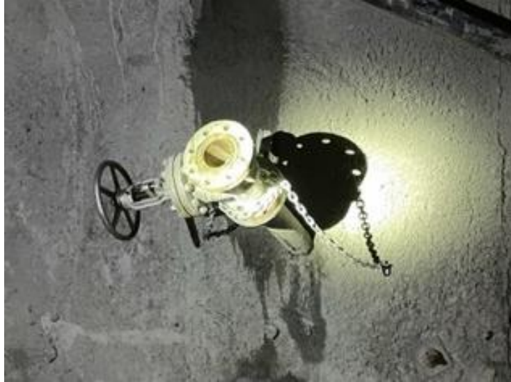
Figure 13: Gate Valve on Standpipe
