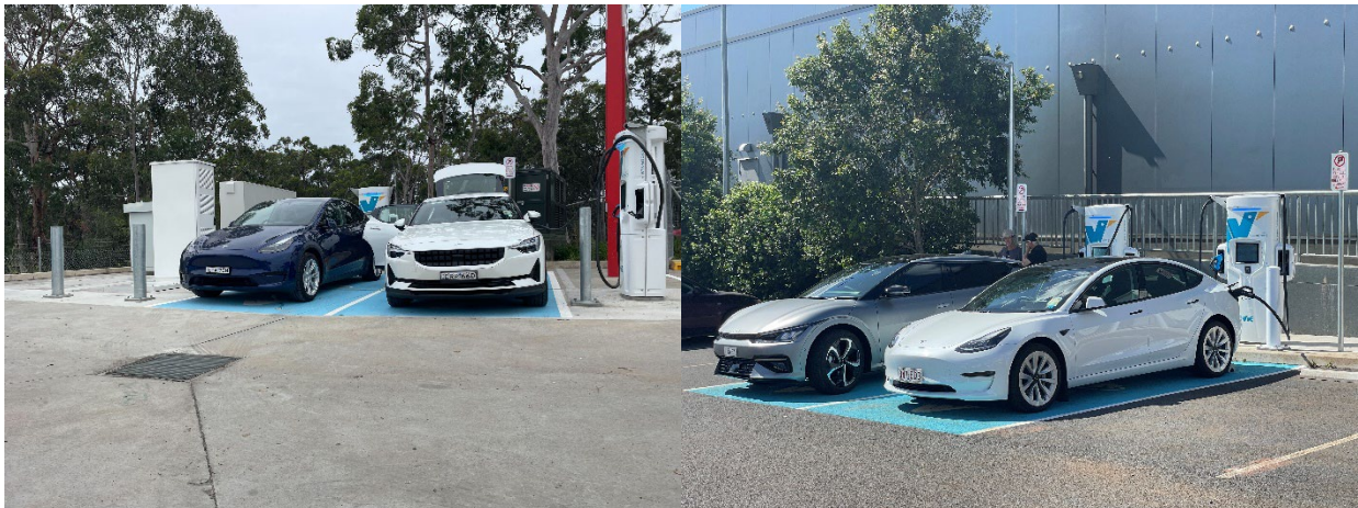
Figure 1: New Evie Networks charging sites launched at Cameron Park NSW (left) and Toowoomba QLD (right)
