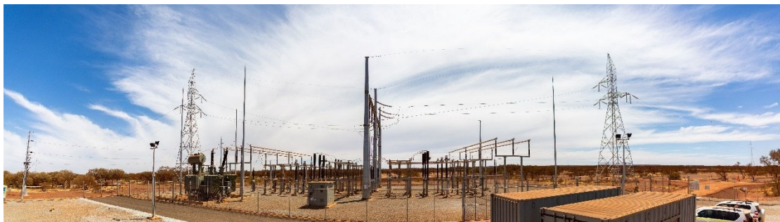
Figure 3: New Christmas Creek Substation
