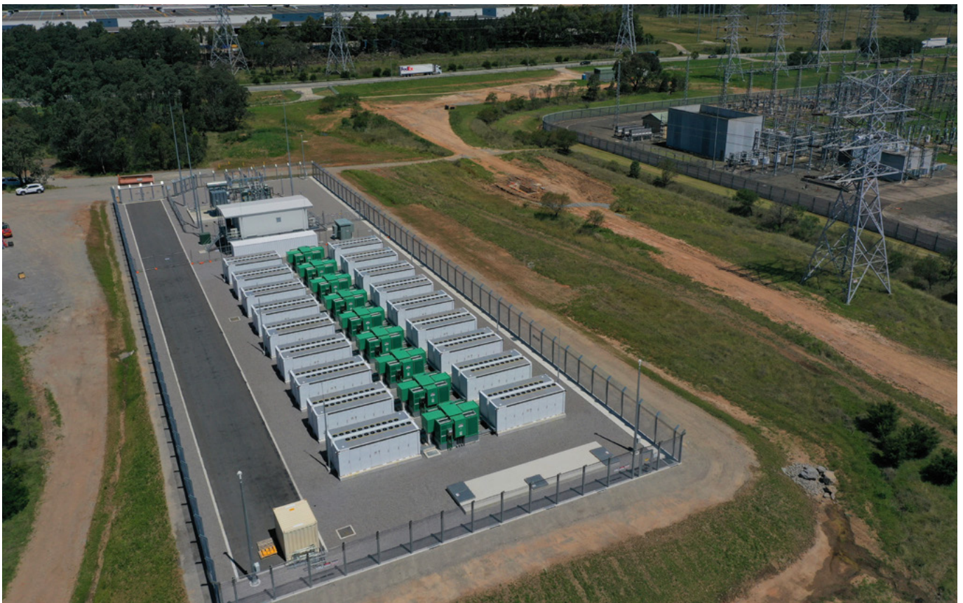
Photo 1 – Wallgrove Grid Battery and Sydney West 330/132kV substation aerial view
