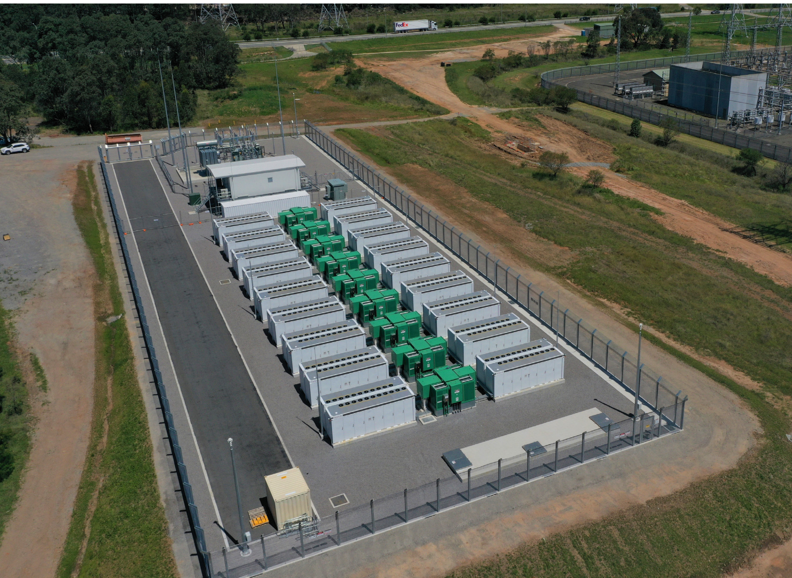
Photo 1 – Wallgrove Grid Battery and Sydney West 330/132kV Substation aerial view
