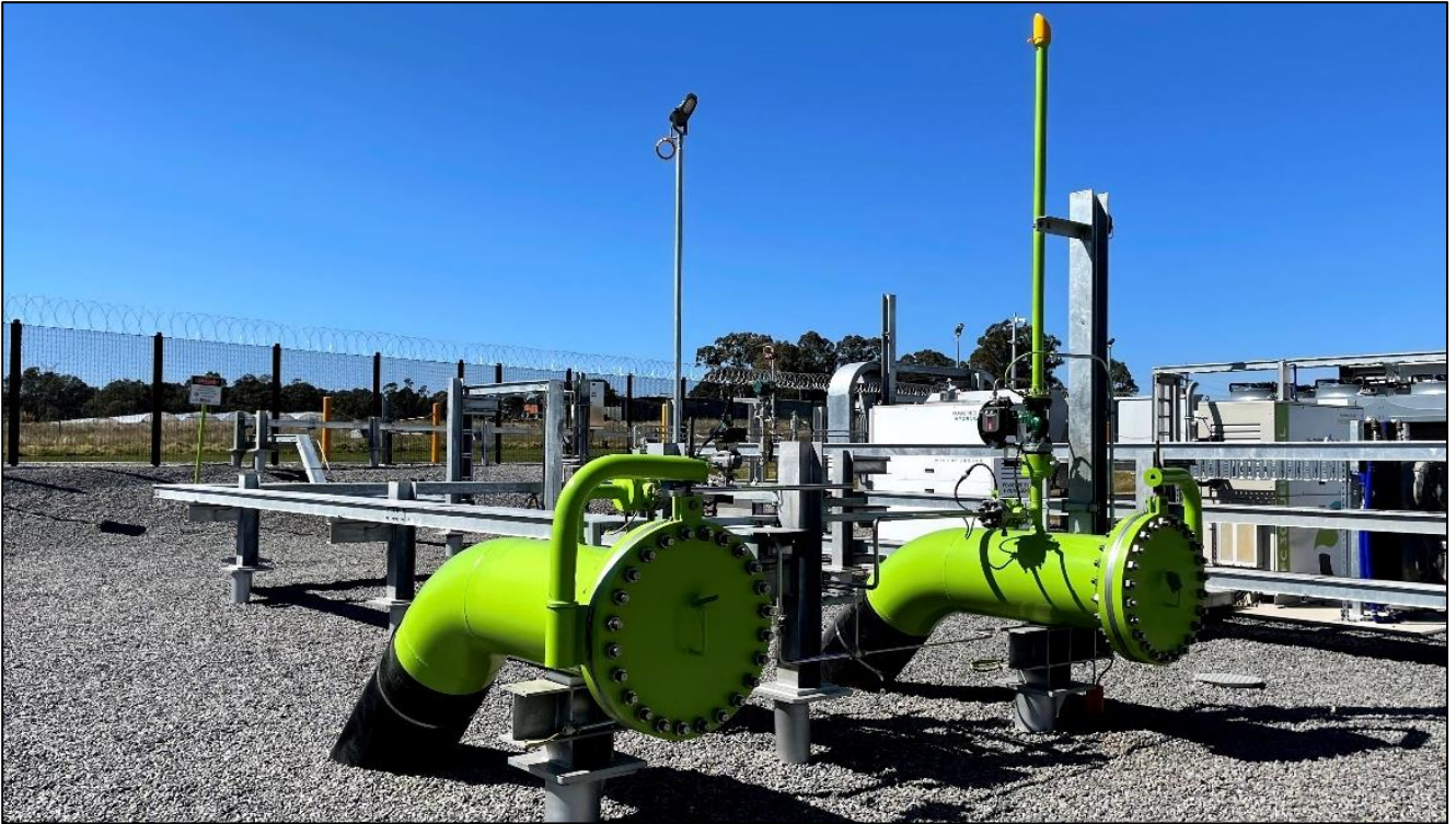
Figure 7: WSGHH hydrogen storage pipeline (buffer store).
