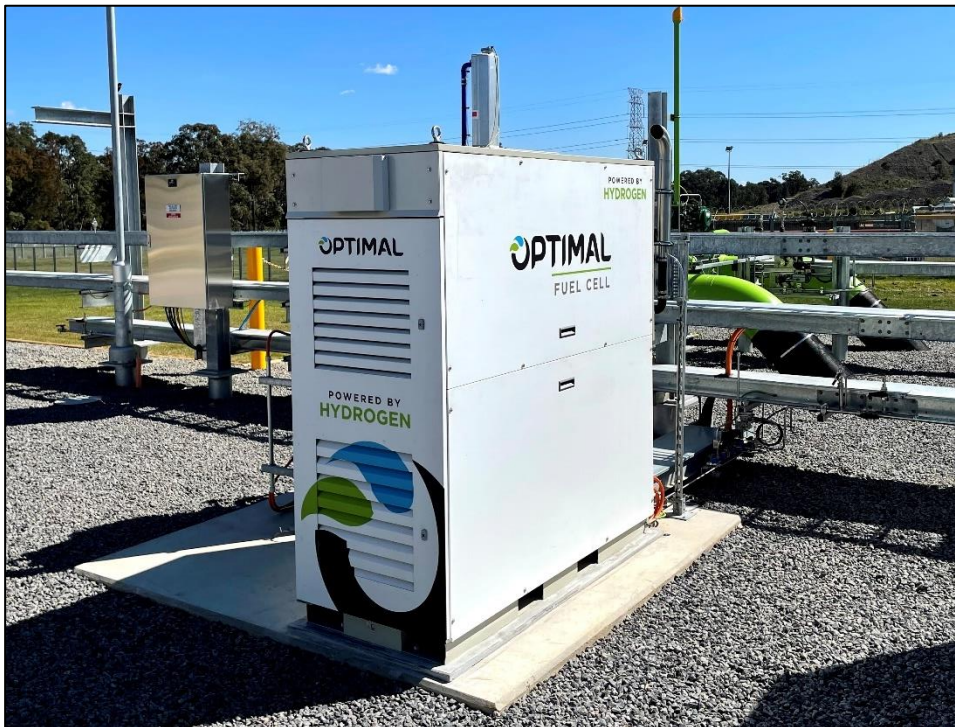
Figure 14: The 35 kW hydrogen fuel cell at the WSGHH.
