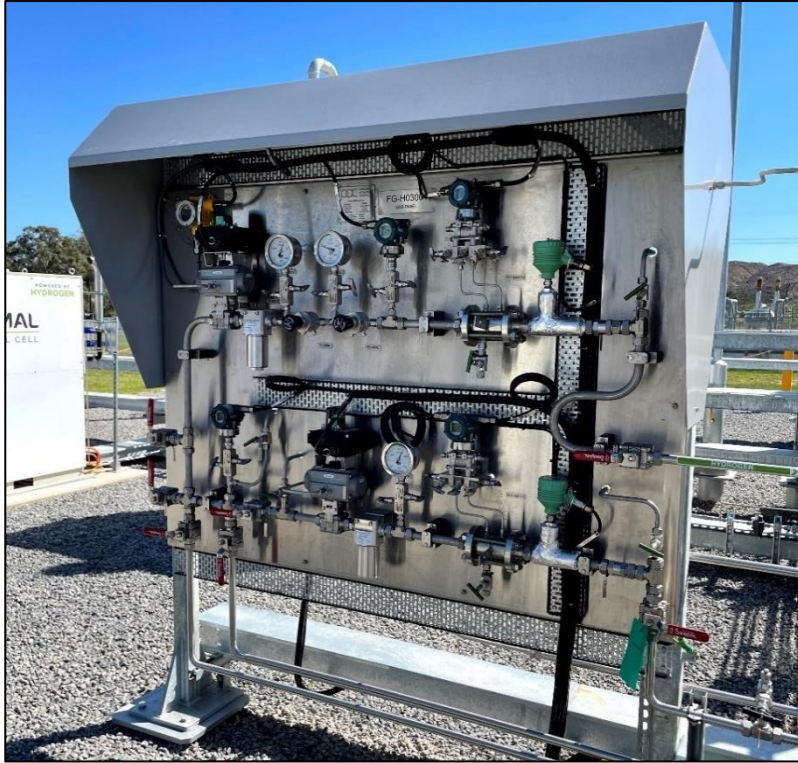
Figure 12: The gas panel package at the WSGHH.
