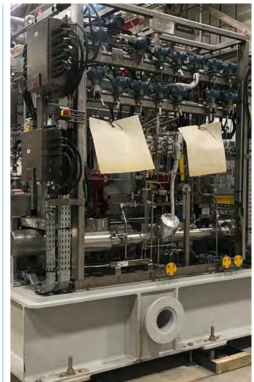
| Main Compressor Skid - sCO 2 STEP Demo - GTI
