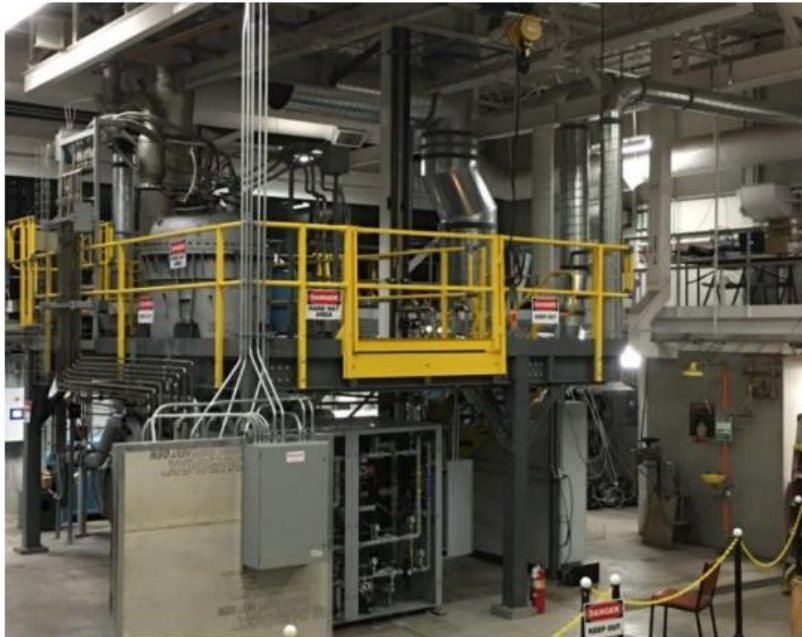
Figure 31 Pilot plant flash reactor (8)
