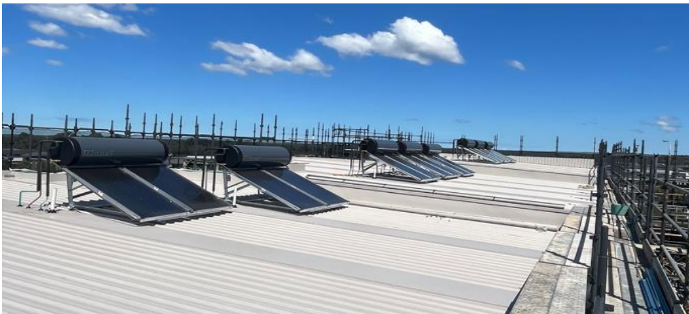
Figure 1. Solar hot water units on a rooftop.
