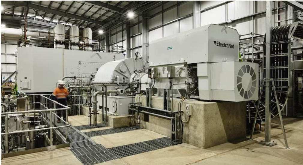
Figure 4 – Synchronous Condenser (Source: Electranet)
