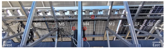
Figure PP4.5.1: The rear view of the outdoor convective measurement setup. The placement of the temperature sensor are indicated on module M4 in the red circle. Module M3 and M4 have aluminium and 3D-printed polymer VGs attached to the backsheet.
