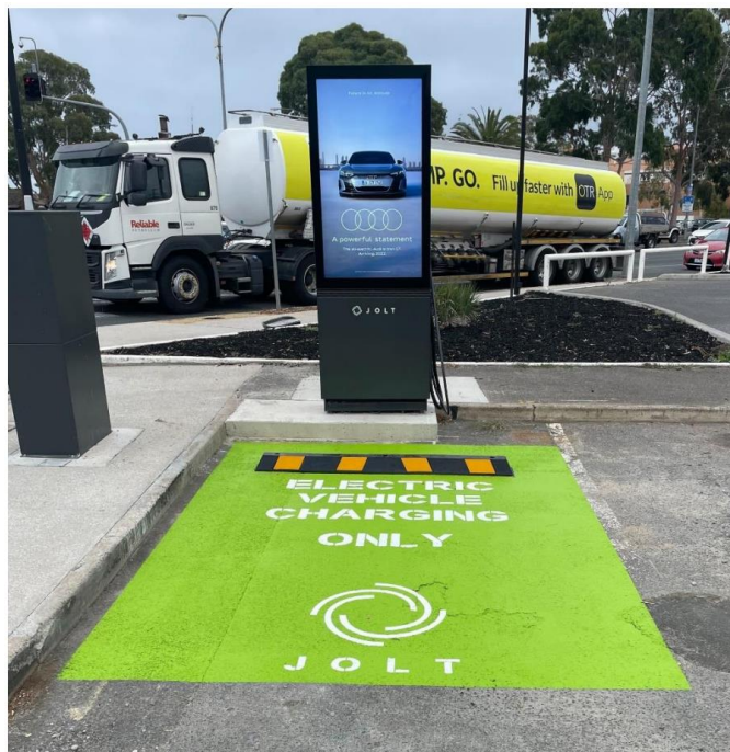
Figure 17 – JOLT Charging Bay Markings
