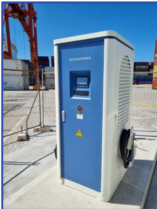
Figure 4: Installation of 260kW Dual Port Charger at Patrick Terminals Fremantle
