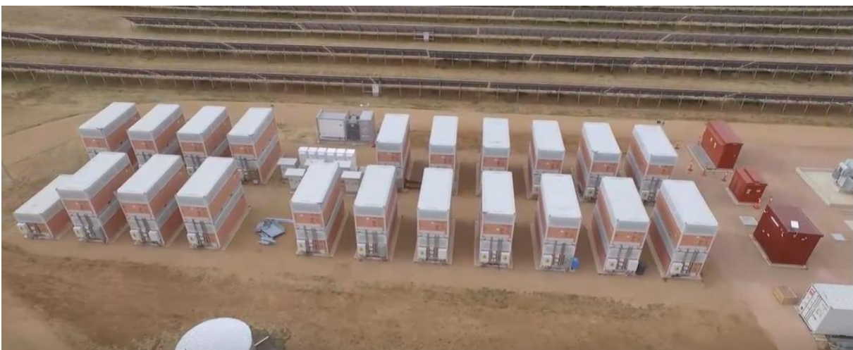
Figure 1: Aerial view of the Yadlamalka Vanadium Flow Batteries
