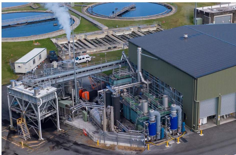
Figure 1: Loganholme WWTP Permanent Gasification Facility
