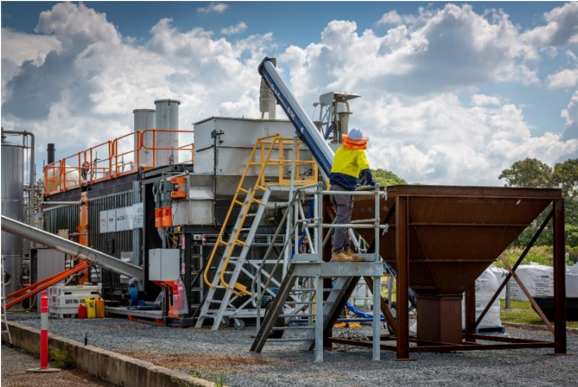
Figure 2: Loganholme WWTP Demonstration Plant
