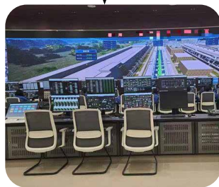
Poly-Si plant control room
